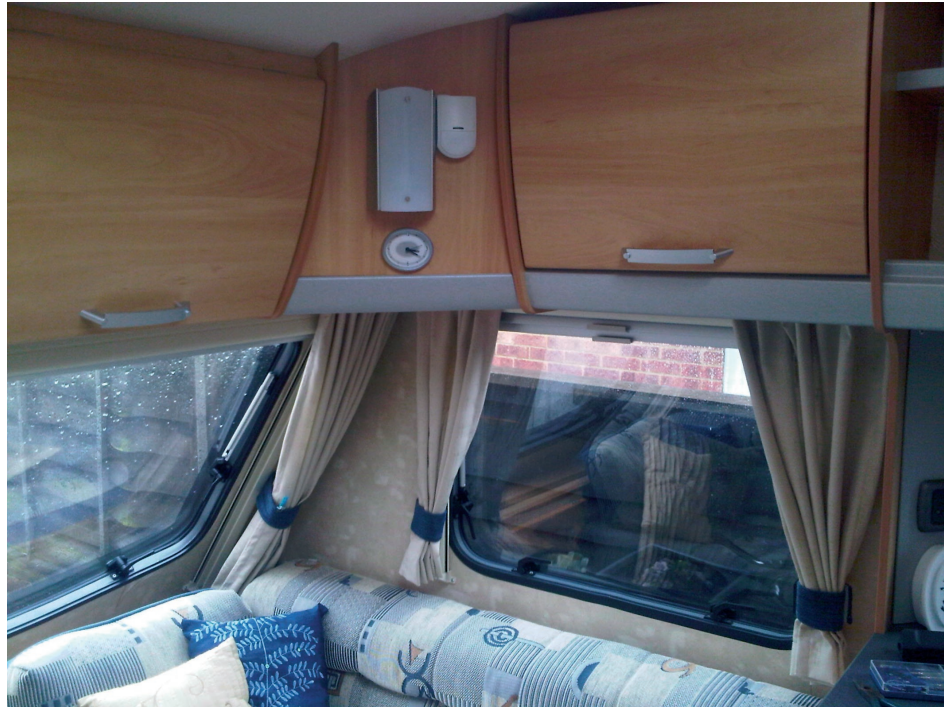
PIR Installed to right of light. RMC300R and siren installed behind panelling
